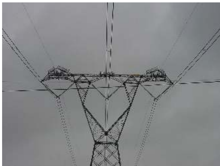
Comprehensive fitting strategy as implemented on the Hendrina-Kriel 400kV line
