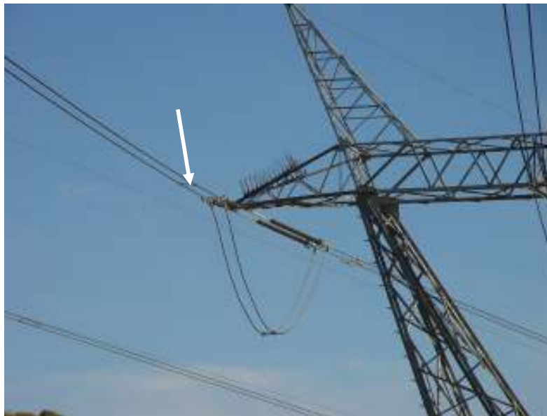
Picture of incorrect fitting leaving the landing plates exposed
